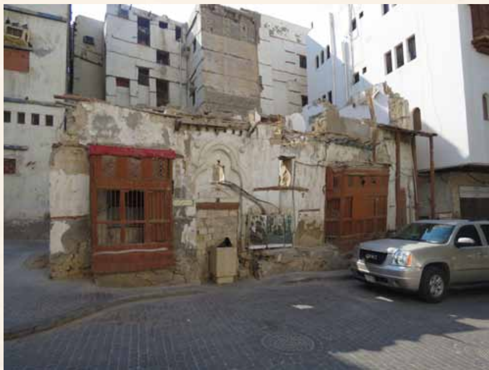
Crown Prince Project to Save and Consolidate the Historic, Archaeologic and National Listed Buildings in Historic Jeddah (56 historic buildings) Bayt Ferwan
