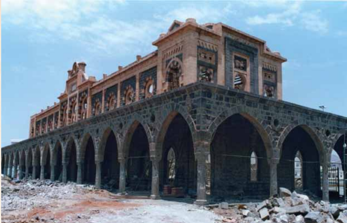
The main building of the Hijaz Railway station during restoration - Al-Madina Al-Munawara
