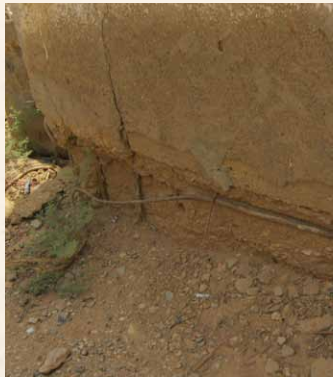
Al Murih Mosque damaged concrete bases armed-Arriyadh
