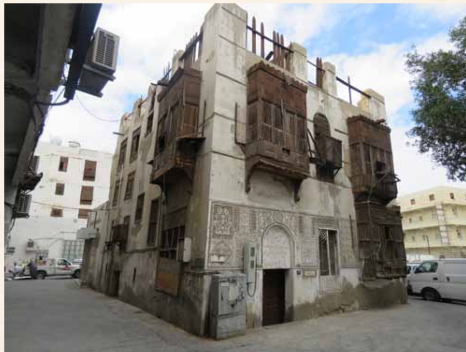
Crown Prince Project to Save and Consolidate the Historic, Archaeologic and National Listed Buildings in Historic Jeddah (56 historic buildings) Bayt Hazuqua
