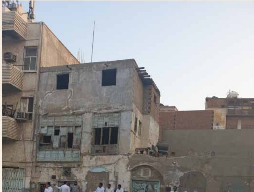
Crown Prince Project to Save and Consolidate the Historic, Archaeologic and National Listed Buildings in Historic Jeddah (56 historic buildings) Ribat Al Sumal
