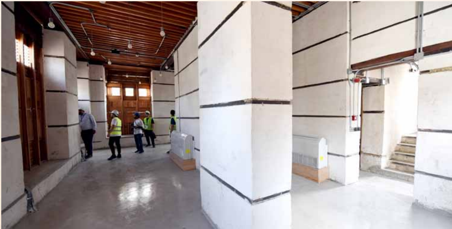
Study, consolidation and restoration of Jeddah's high-risk historic buildings - Daffa House- Historic Jeddah
