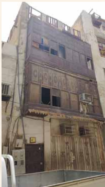
A Project to Prepare a Building Information Modeling System for Historic Buildings (HBIM) in the Historic Jeddah District (For 100 Buildings) N° 1276
