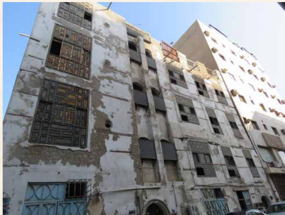
Crown Prince Project to Save and Consolidate the Historic, Archaeologic and National Listed Buildings in Historic Jeddah (56 historic buildings) Shokri
