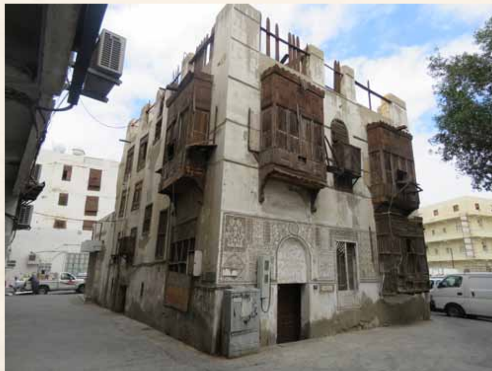
A Project to Prepare a Building Information Modeling System for Historic Buildings (HBIM) in the Historic Jeddah District (For 100 Buildings) Bayt Hazuqua
