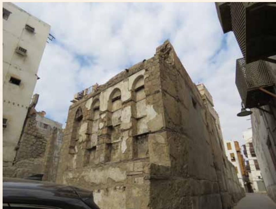
Crown Prince Project to Save and Consolidate the Historic, Archaeologic and National Listed Buildings in Historic Jeddah (56 historic buildings) Bayt Shahat
