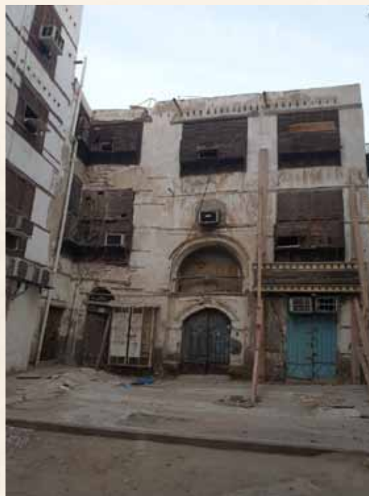
Crown Prince Project to Save and Consolidate the Historic, Archaeologic and National Listed Buildings in Historic Jeddah (56 historic buildings) Waqaf Falah School
