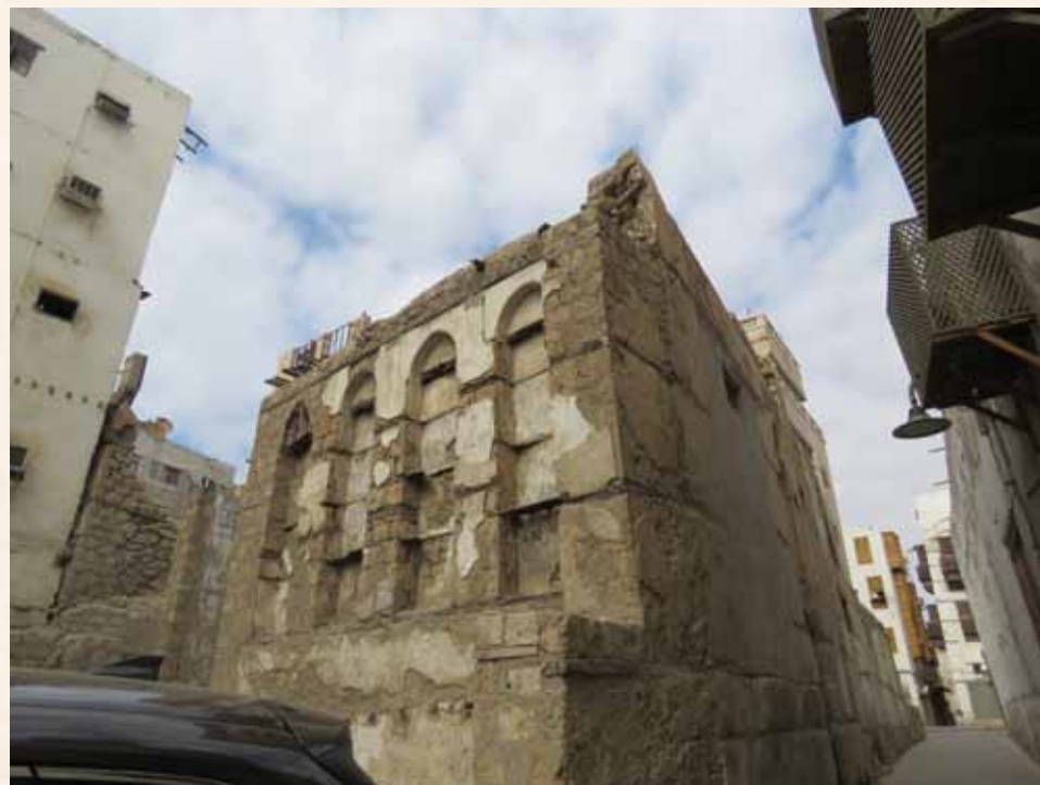
A Project to Prepare a Building Information Modeling System for Historic Buildings (HBIM) in the Historic Jeddah District (For 100 Buildings) Bayt Shahat
