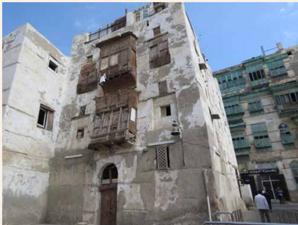
Crown Prince Project to Save and Consolidate the Historic, Archaeologic and National Listed Buildings in Historic Jeddah (56 historic buildings) Waqaf Shafi Sagheer
