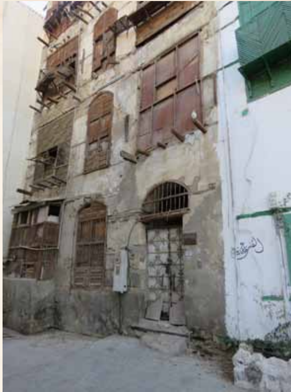
Crown Prince Project to Save and Consolidate the Historic, Archaeologic and National Listed Buildings in Historic Jeddah (56 historic buildings) Bayt Al Jifri
