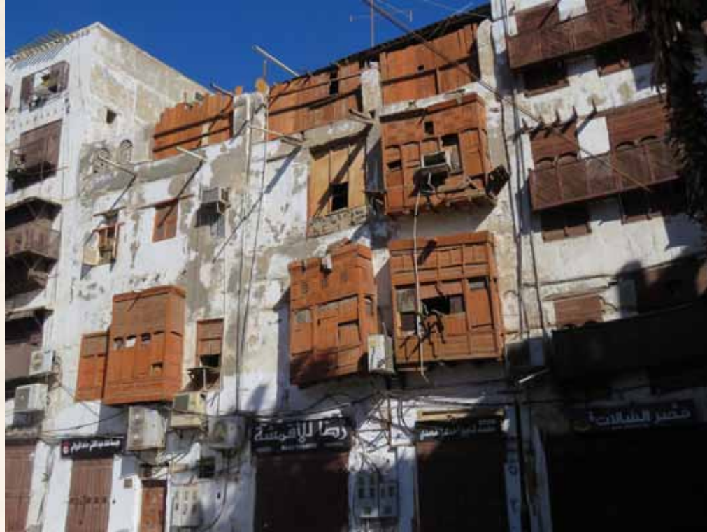
Crown Prince Project to Save and Consolidate the Historic, Archaeologic and National Listed Buildings in Historic Jeddah (56 historic buildings) Abed
