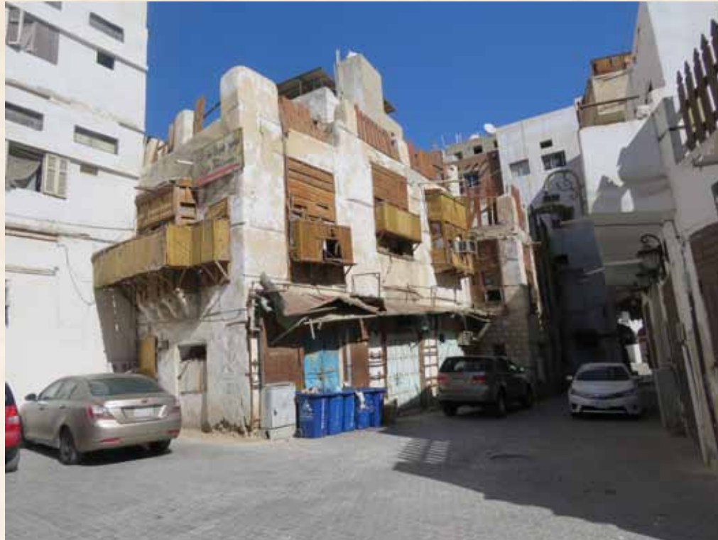
Crown Prince Project to Save and Consolidate the Historic, Archaeologic and National Listed Buildings in Historic Jeddah (56 historic buildings) Waqaf Nassif
