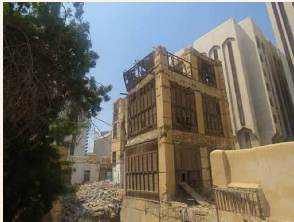
Crown Prince Project to Save and Consolidate the Historic, Archaeologic and National Listed Buildings in Historic Jeddah (56 historic buildings) Banajah Palace
