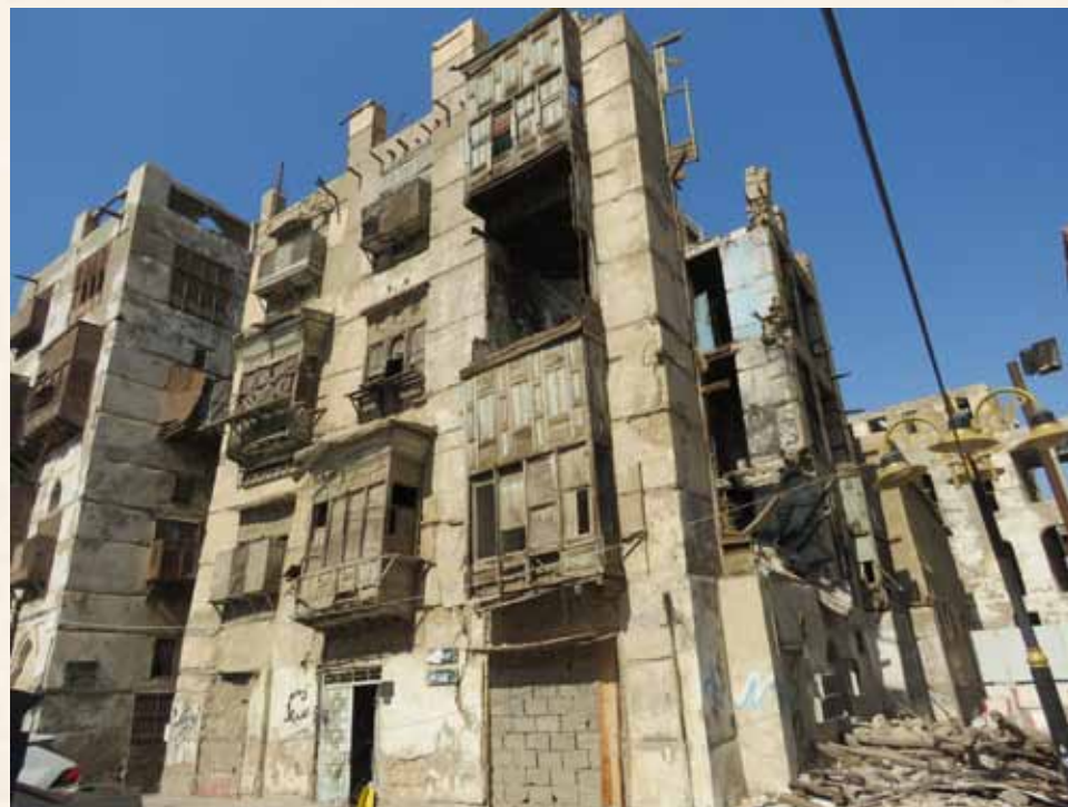
Crown Prince Project to Save and Consolidate the Historic, Archaeologic and National Listed Buildings in Historic Jeddah (56 historic buildings) Ribat Al-Hindi
