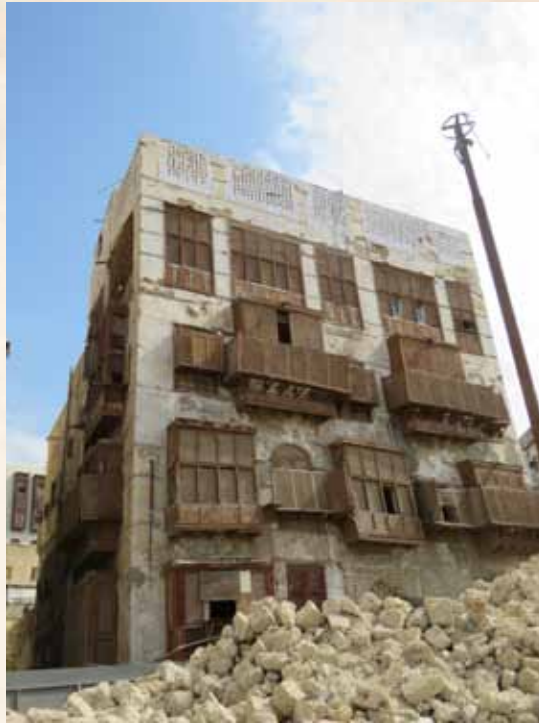
Crown Prince Project to Save and Consolidate the Historic, Archaeologic and National Listed Buildings in Historic Jeddah (56 historic buildings) Abdullatif banajah
