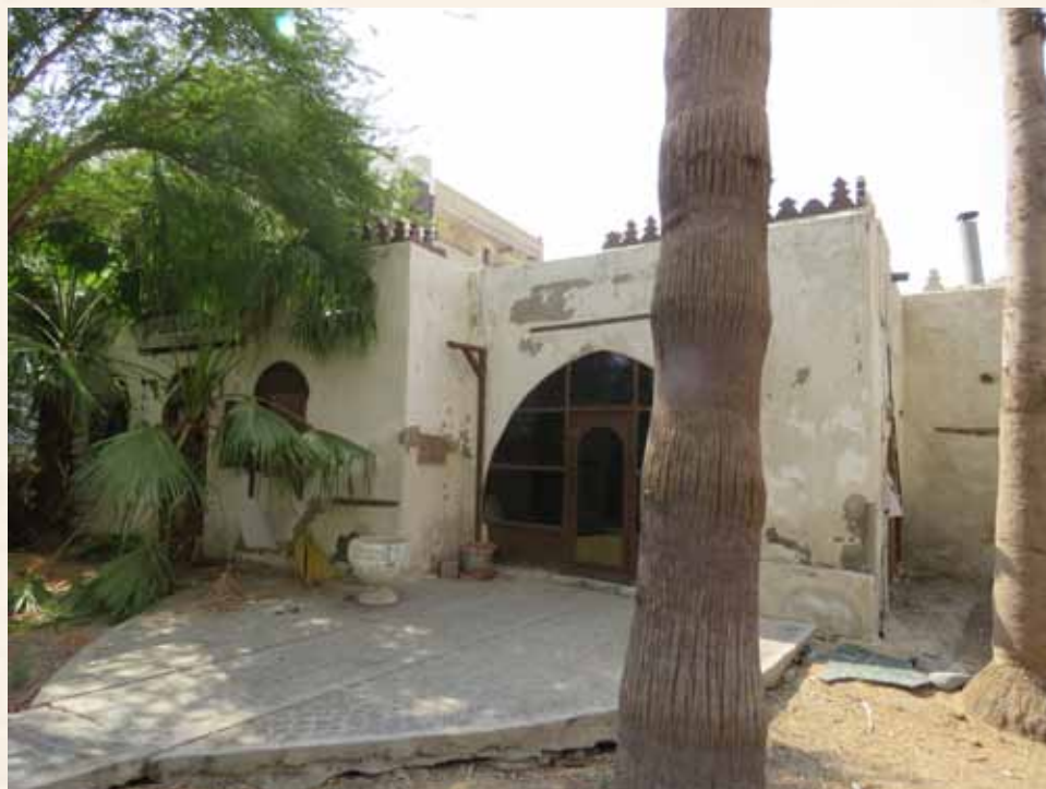
Crown Prince Project to Save and Consolidate the Historic, Archaeologic and National Listed Buildings in Historic Jeddah (56 historic buildings) Bayt Al Kuttab
