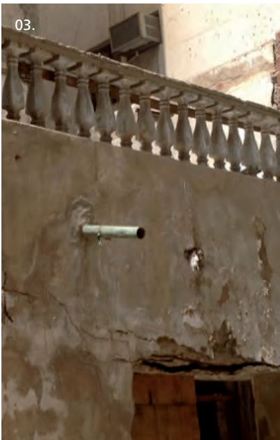
03_ Gargoyle used for the rainwater runoff from the terraces of a building in Jeddah.
