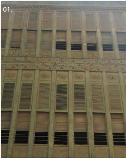
01_02 Wooden elements that characterize and decor the traditional buildings facades in Jeddah.
